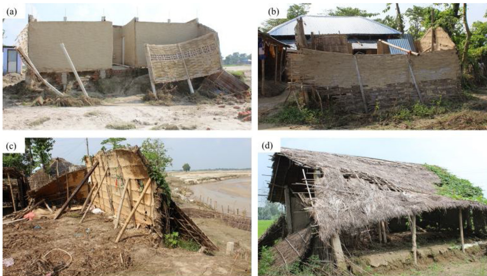
Fig. 4. a) Wattle and daub house partly damaged by flood, b) a destroyed wattle and daub house restored for temporary use, c) remains of a building (one wall) as three other walls were destroyed by the flood, d) a distorted wattle and daub house with collapsed and washed away walls.
