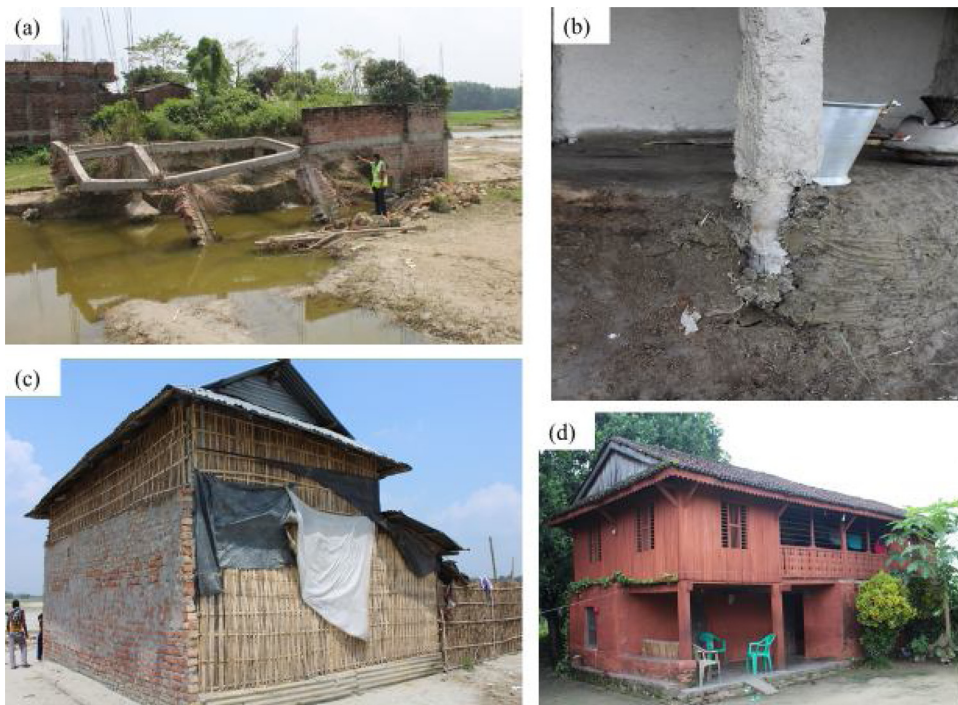
Fig. 5. a) A washed away under-construction reinforced concrete building, b) ejected concrete pole displays the marginal depth of insertion to the ground, c) single wythed brick wall construction in the direction perpendicular to likely flood direction, d) vernacular multi-wythed flood resilient construction practice in southern Nepal.
